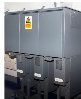
SS 3 2 x Merlin Gerin SE6 SF 6 Switches and Circuit Breaker
