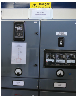
Live Phasing Demonstration Rig 2 x Rayrolle LMT23 OCB
